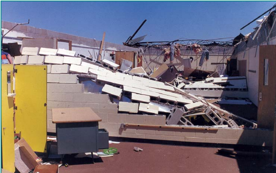
Figure 3-17 Interior and exterior unreinforced masonry walls were damaged when reinforced bond beams failed.
