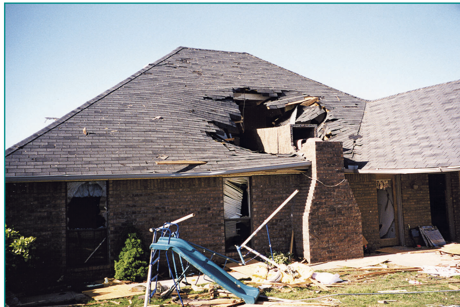
Figure 4-3 Failure of brick chimney under tornado winds damaged the room of this house in Moore, Oklahoma.
