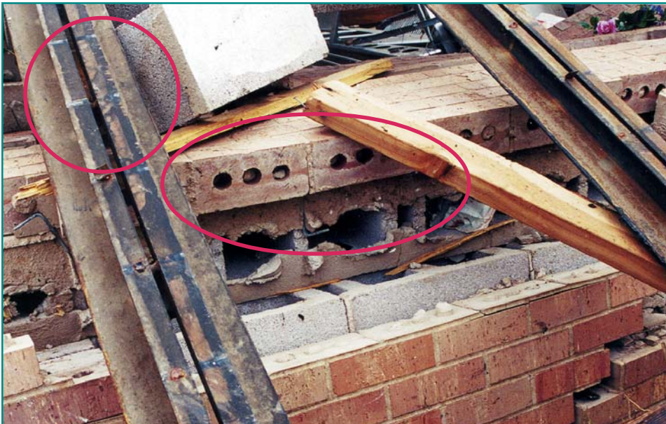
Figure 3-21 Failed roof structure showing broken welds between metal roof deck and tops of joists (upper circle) and lack of vertical reinforcement (bottom circle).
