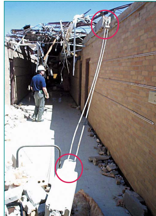
Figure 3-18 Corridor area. Separation of reinforced bond beam (indicated by circles) from supporting wall.
