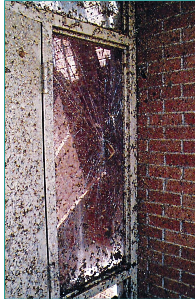
Figure 3-22 Impact performance of laminated glass. The corner of a table penetrated this laminated glass window, but the glass remained in its frame.
