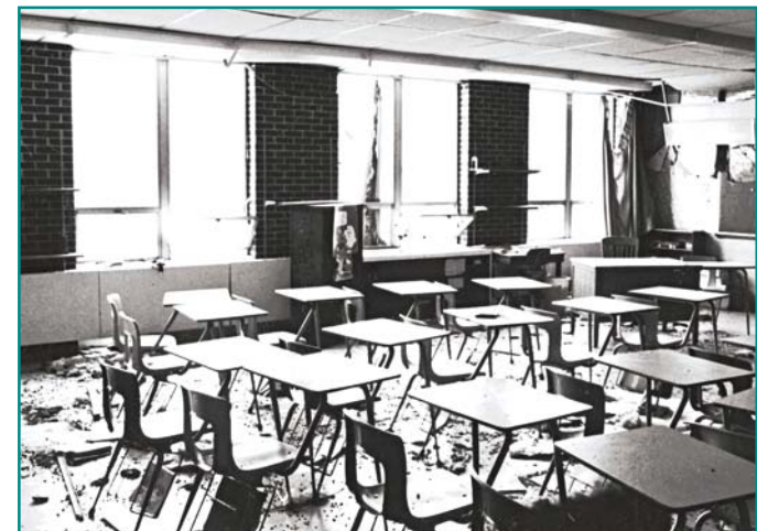
Figure 3-11 Broken windows and debris in classroom of St. Augustine Elementary School building.
