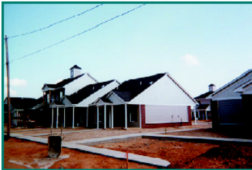
In Arkadelphia, USDA Rural Development Administration funds were used to build attractive low-income, multi-family units.
