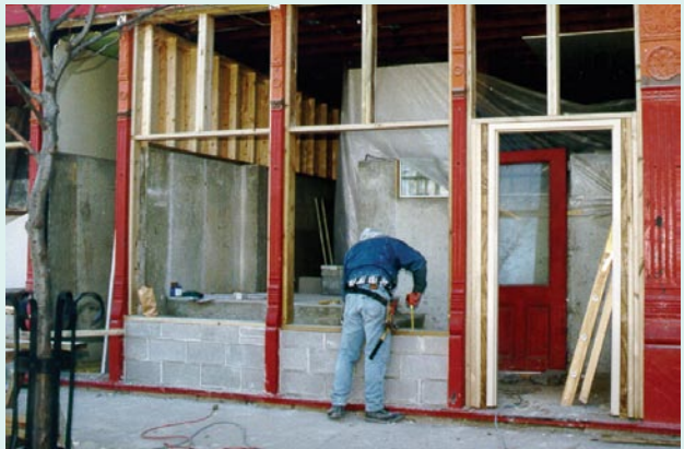
Top: Restored and retrofitted building. Middle: To provide additional protection against floodwater, removable watertight floodgates were incorporated into the buildings. Bottom: Floodproofing in action in Darlington, Wisconsin.
