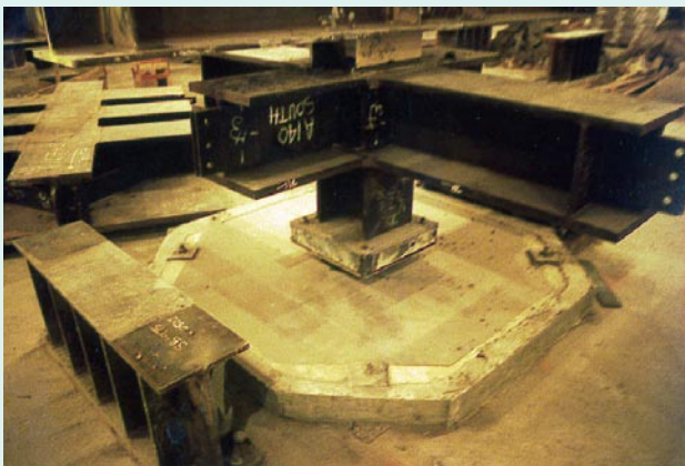
San Francisco City Hall Base Isolation System.
